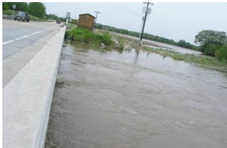
Figure 1.1 Partially inundated bridge deck at Salt Creek, NE.
